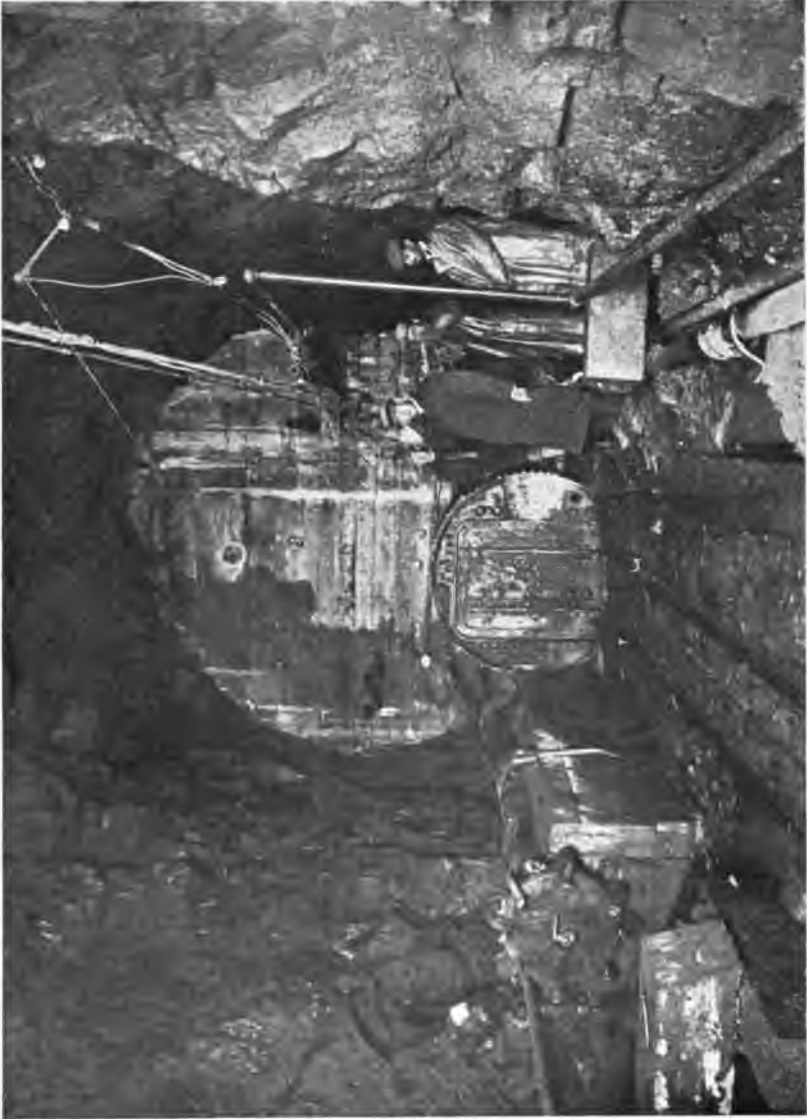
PLATE 189. —Eastview Tunnel Concrete Bulkhead, Material and Timber Locks for Compressed Air Section.
